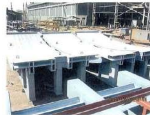
Settler Flash Furnace: Bottom Saddle (109.380 kg)
