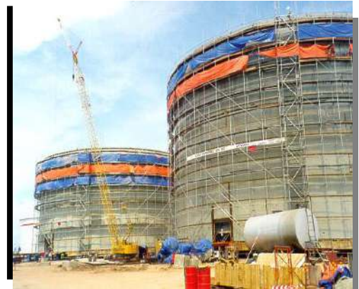
PETROCHEMICAL STORAGE TANKS
