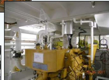
Auxiliary engine room
